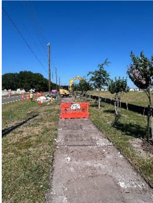
Const Package 4B Prepping for Pipe Installation Old Bartow Lake Wales Road
